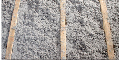
Cellulose insulation level on 2x6 ceiling joists yeilds an R-Value of approximaltey 20. This is not enough. FEC can help you get to at least R30
