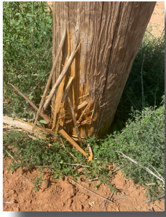
Damaged pole found in a freshly plowed field
